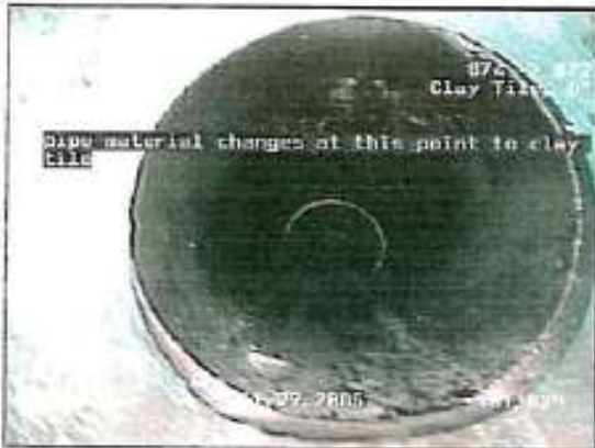
IMAGE: 11a, TAPE #: 11/29/2005 101.2FT, pipe material changes at this point to clay tile
