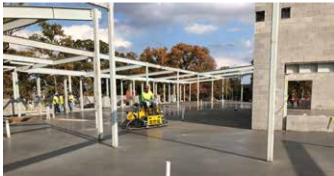
Pad site for the Animal Services and Adoption Center. The facility was funded through a voter approved bond.
