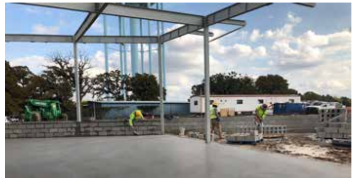
Structural steel framing has been completed for the new Animal Services and Adoption Center located off TCC Rd.
